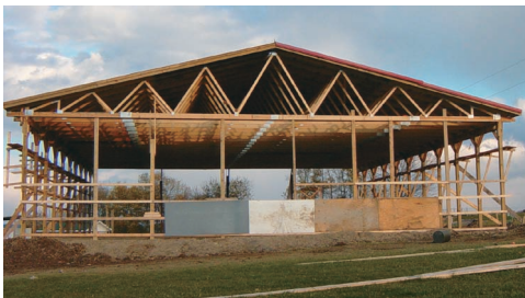
Photo 6.3 Because roof trusses, such as those shown, require support only at their ends, it is possible to construct buildings with large, unobstructed floor areas.
