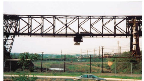
Photo 6.2 Two K trusses were used as the main components of the movable bridge shown which moved above a large stockpile of ore. The bucket below the trusses picked up ore and redeposited it until the ore was thoroughly mixed. The ore was then sent to the mill for processing into steel.
